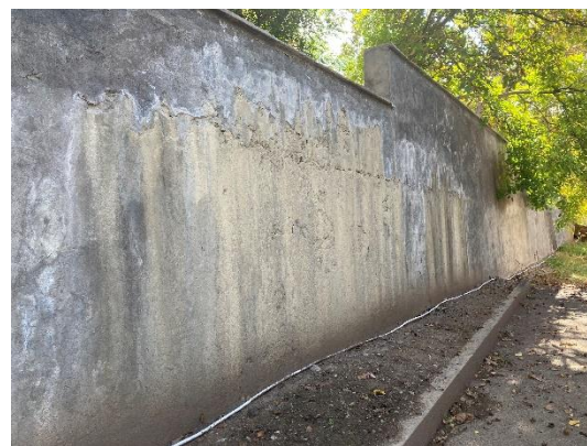
Outer wall of Malishka Kindergarten damaged by constant water leakage from the drainage
