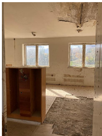
Deteriorated block of building to be renovated
