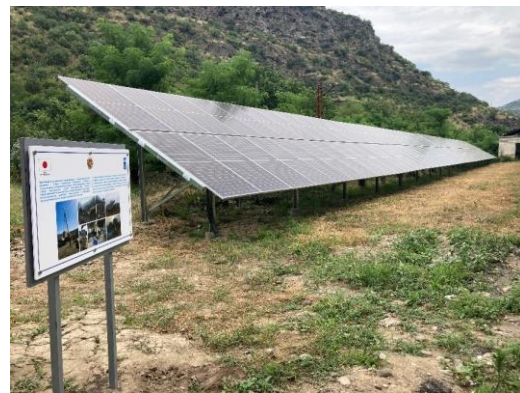
Installed photovoltaic station
